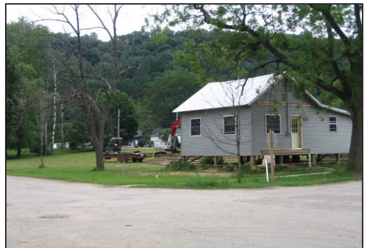
Diagonally across the street from the Evans home, a neighbor is preparing to build a new, elevated foundation next to his house to lift it above the Base Flood Elevation. It was already raised on 4x4 timbers, ready for moving, when the June storm of 2008 arrived, thus avoiding flood damage.
